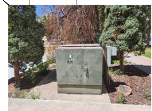
EXISTING IDAHO POWER TRANSFORMER TO REMAIN
